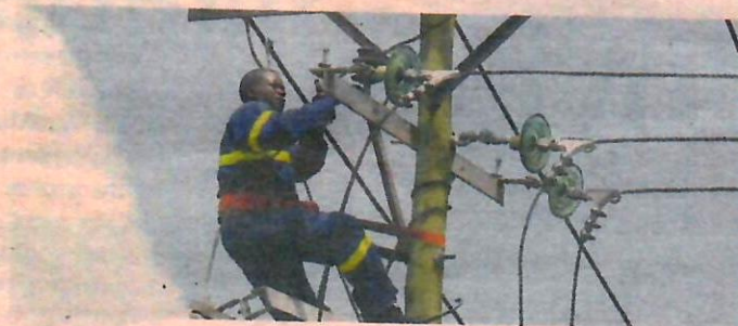
COMPETITION A Kenya Power technician fixes a transmission line in Nairobi. –FILE
